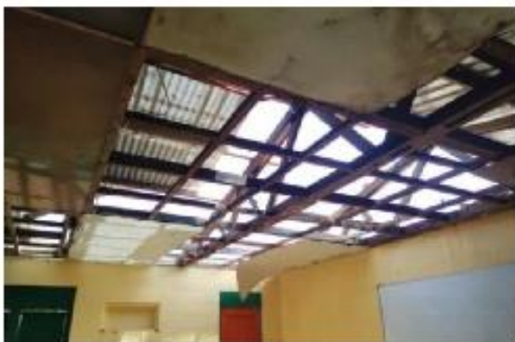
Onesua College – Damage to Junior Science Lab
